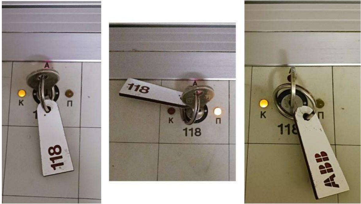
Figure 46. Detail of the three-position key for handling switches 118 on the Larissa Control Panel.
