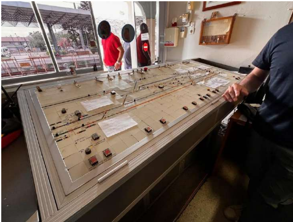
Figure 37. The control panel at Larissa Station
