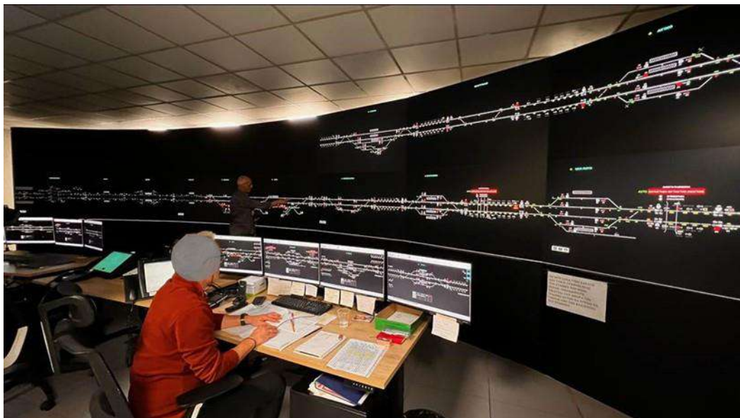
Figure 52. Digitalised traffic control room in Larissa station, with experienced staff, in 2025.
